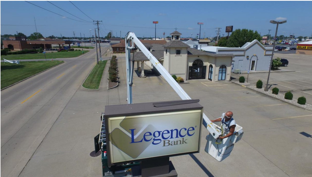
PHOTO #3, Legence Bank Mt. Vernon sign:
